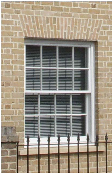
Traditional timber sash window to a new house set 100mm back from face of the brickwork and with a sub-cill. Note also the use of Flemish bond in the brickwork together with the shaped 'voussoir' bricks over the opening.
